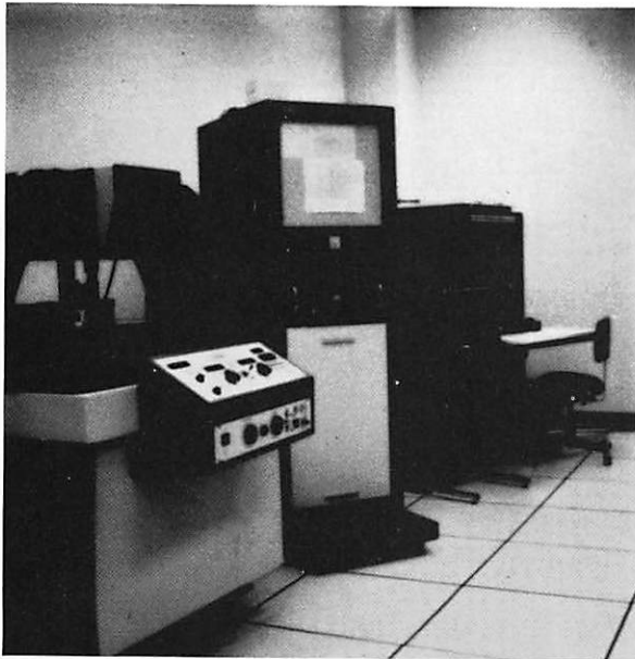
b) Left Hand View of Image Equipment Room
